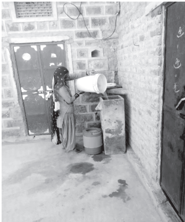
Bio-sand water filter installed in one of the beneficiaries' homes in the Thar region
