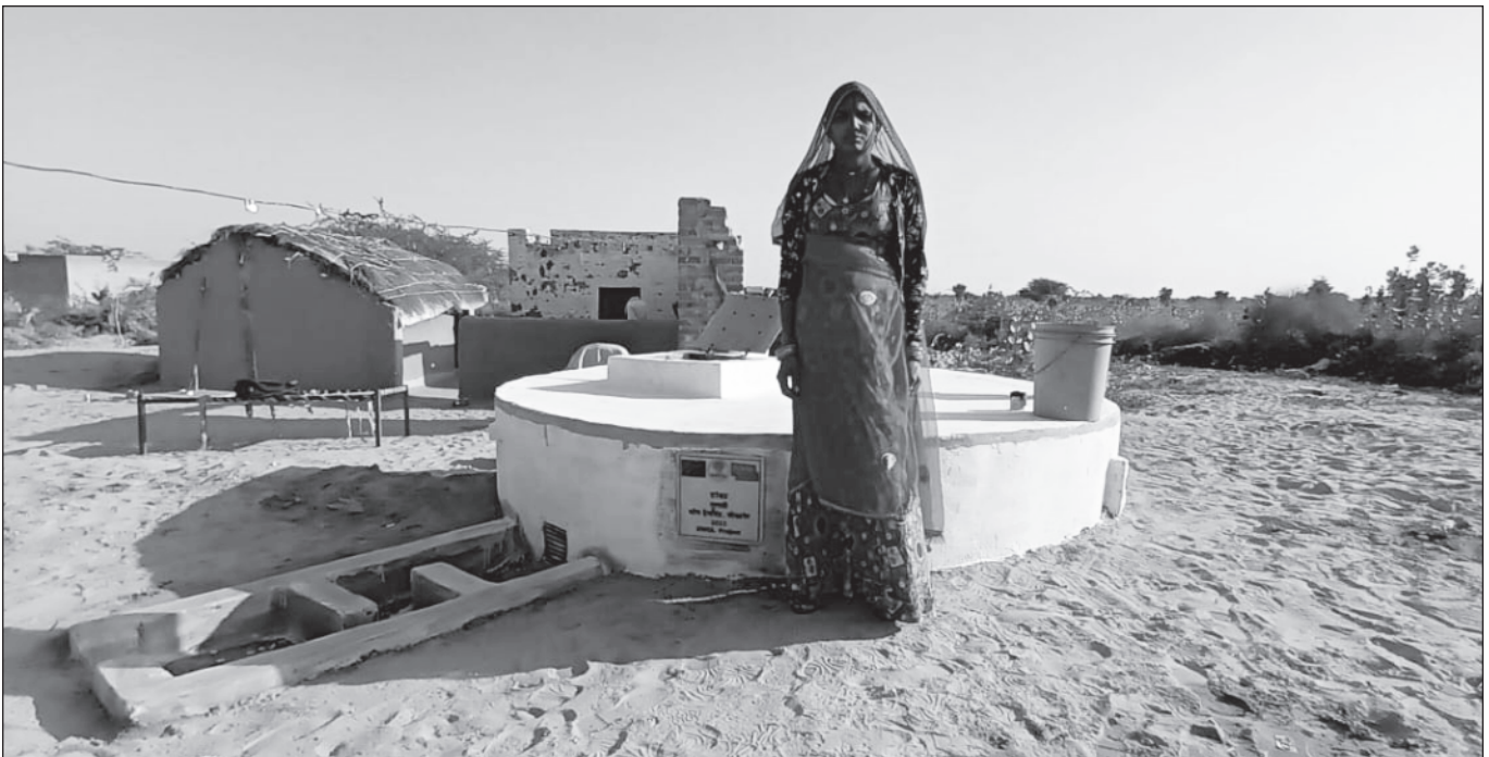
Taanka construction ensuring water security for one of the beneficiaries under the project
